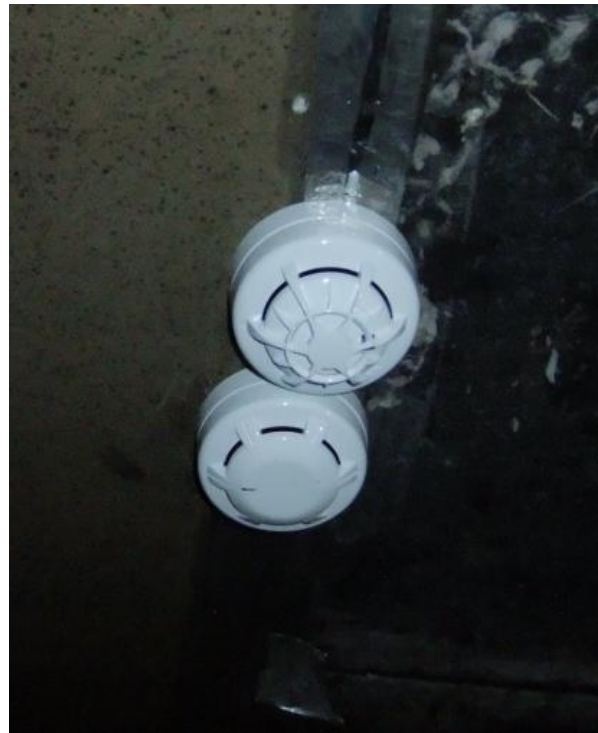
Ceiling mounted optical detectors
