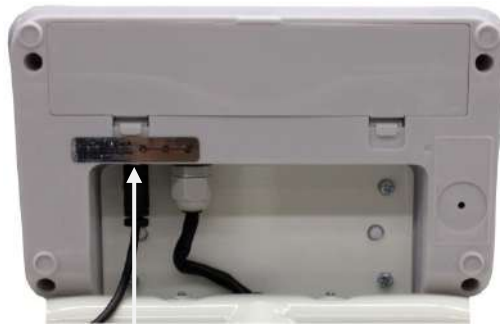
Terminal power supply unit
